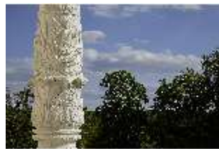
KeBf.I, Strebepfeiler, DI014338, BSV-
